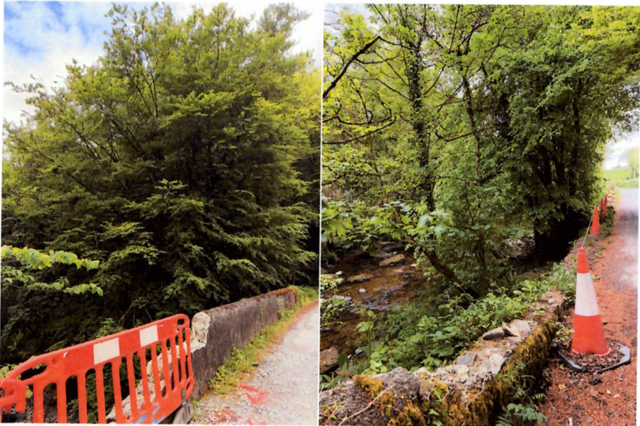
Figure 2. Flood damage at Inchyclough Bridge, showing the watercourse and temporary safety barriers following high water impacts.
